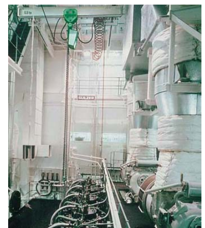
Engine room: JDN Air Hoist PROFI 6 TI in a reel chain trolley
